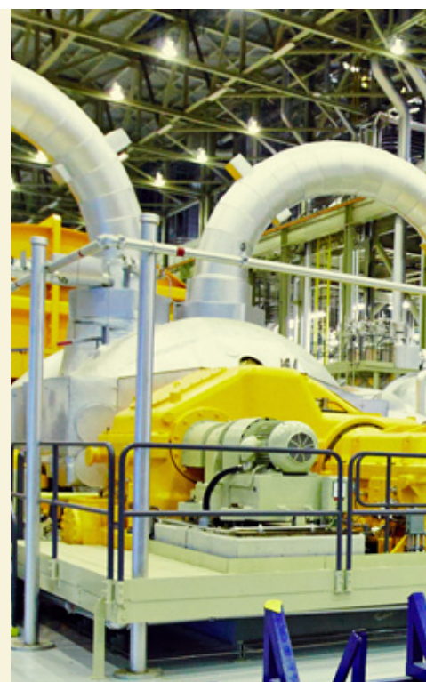
Darlington Nuclear turbine hall.
