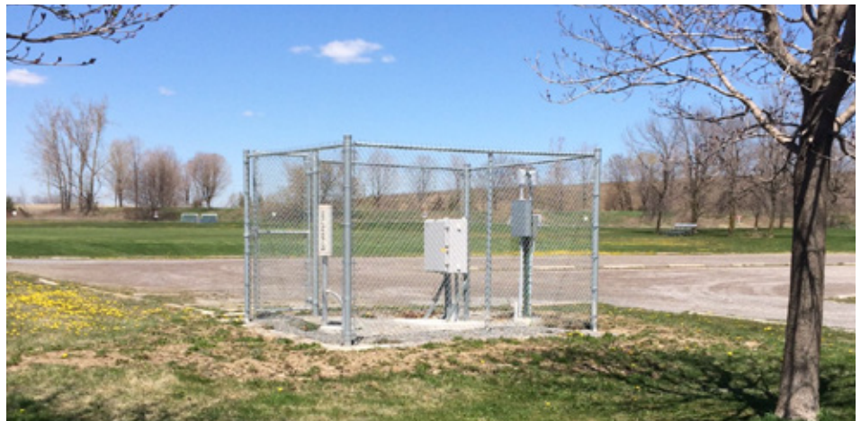
Environmental monitoring station.
