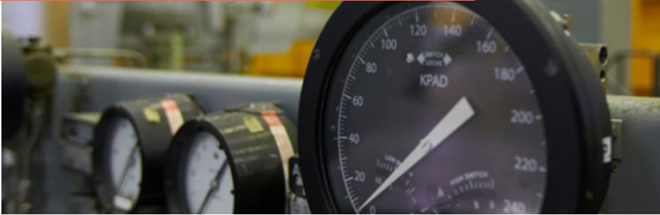
Darlington Nuclear turbine hall.
